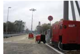
Hydraulic lighting tower, SX-series genset, Enermax 100-kVA generating set
