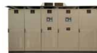
DC&AC UPS 1400A, 42kVA - Ministry of Elect.ty & Water - Kuwait
